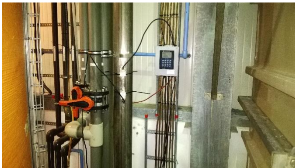
Picture 2-4: Flow measurement of Preox with a portable full pipe flow meter
